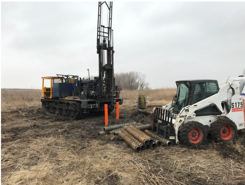
Photo 2-This track-mounted auger rig replaced the truck-mounted rig to better navigate the muddy terrain. This rig operated without issue in the poor site conditions.
