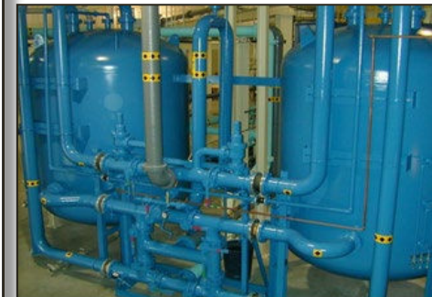
Granular Activated Carbon Treatment Units
