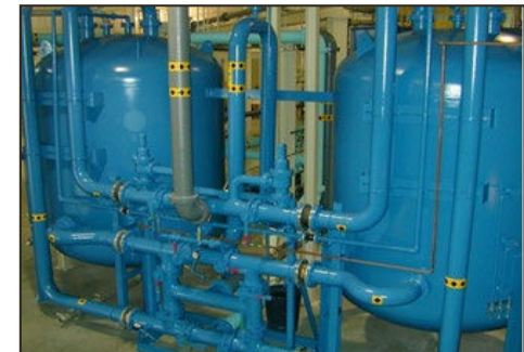
Granular Activated Carbon Treatment Units
